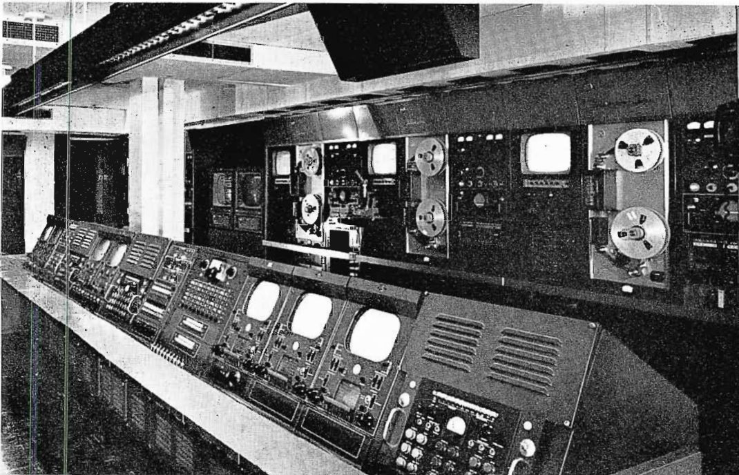
FIG. 9. The camera switching and central control position in the main recording room. From this position all equipments can be started and stopped, monitored and switched.
