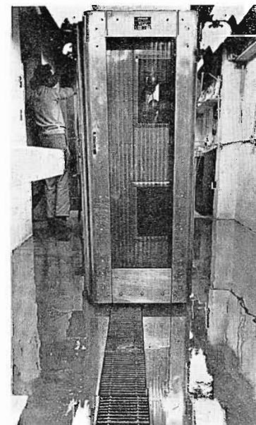
FIG. 60. Note floor drain system beneath film processor.
