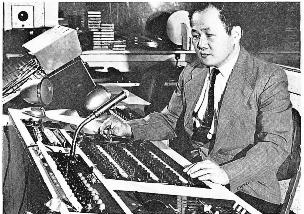
FIG. 2. Studio One control panel containing two special effects banks, two mixing banks, one preview bank and one line bank. Special effects selection panel is also incorporated.
