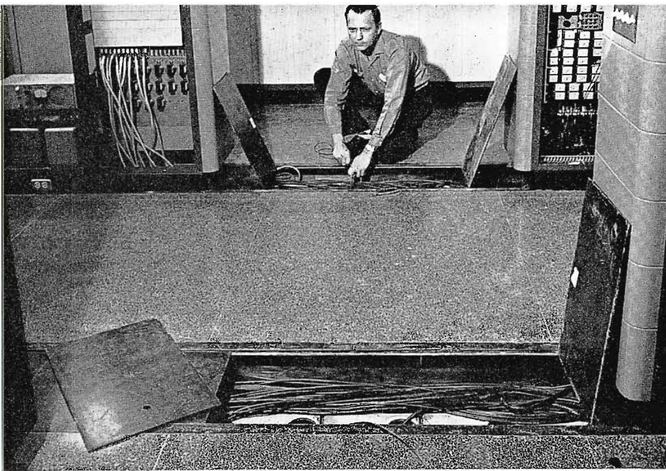
FIG. 29. Don Benedict pulling wire into trenching system. Trenches are under transmitter, consoles, and all racks. All run north and south and are 6 inches deep and 18 inches wide. Since area is designed with cellular metal flooring, cross access trenches are not necessary. Four-inch diameter holes (foreground) lead from trenches into cellular flooring and wires can be pulled down through these holes up into the selected trench.
