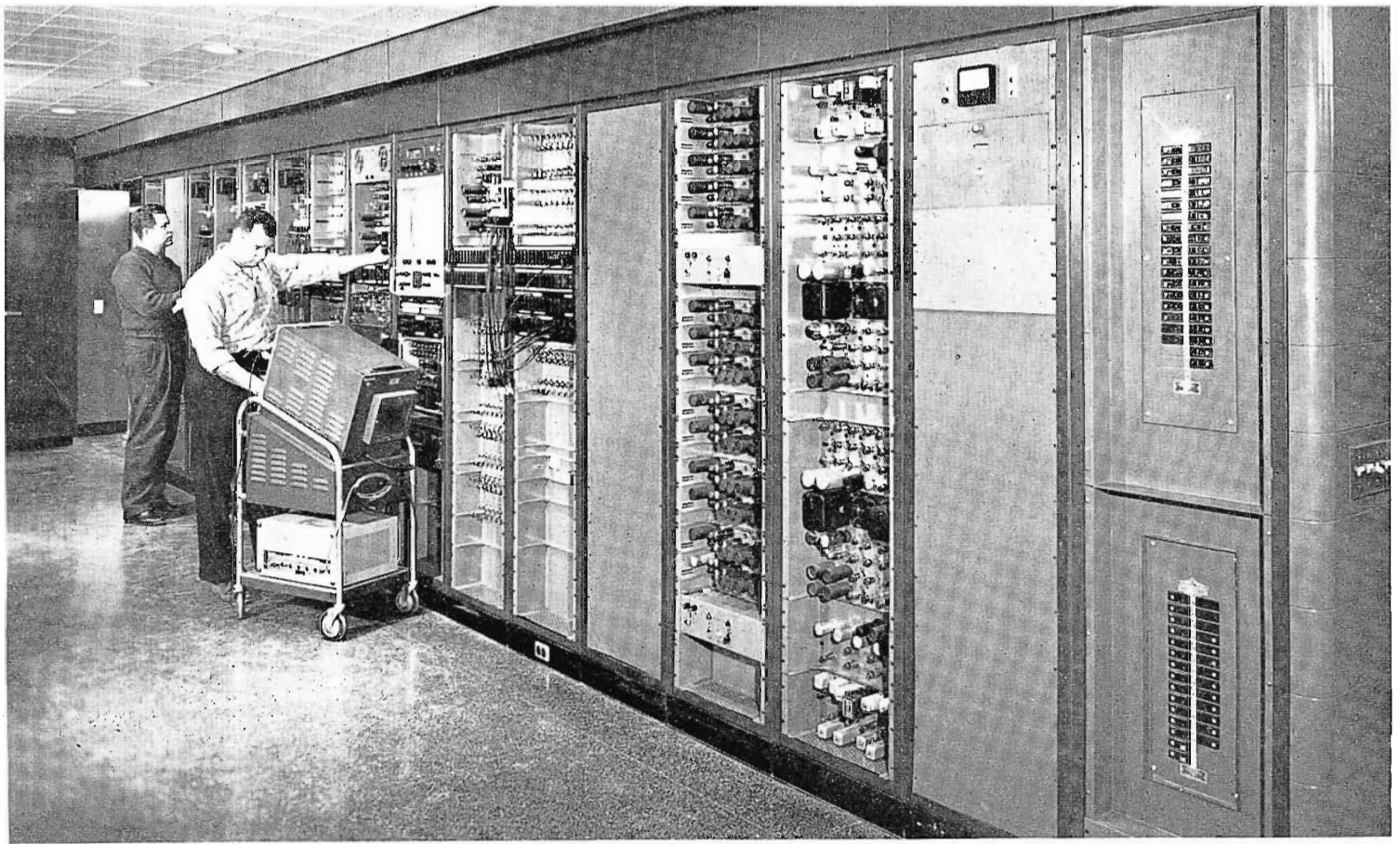
FIG. 33. Clint Barstad and John Reinke, KSTP technicians, at the first row of racks in TV master control. These racks are designated by No. 1 on the far left and ending up with No. 16 on the far right, with No. 16 containing the power distribution. Along the base of all racks power outlets are provided for scopes, voltmeters, tube checkers, etc.
